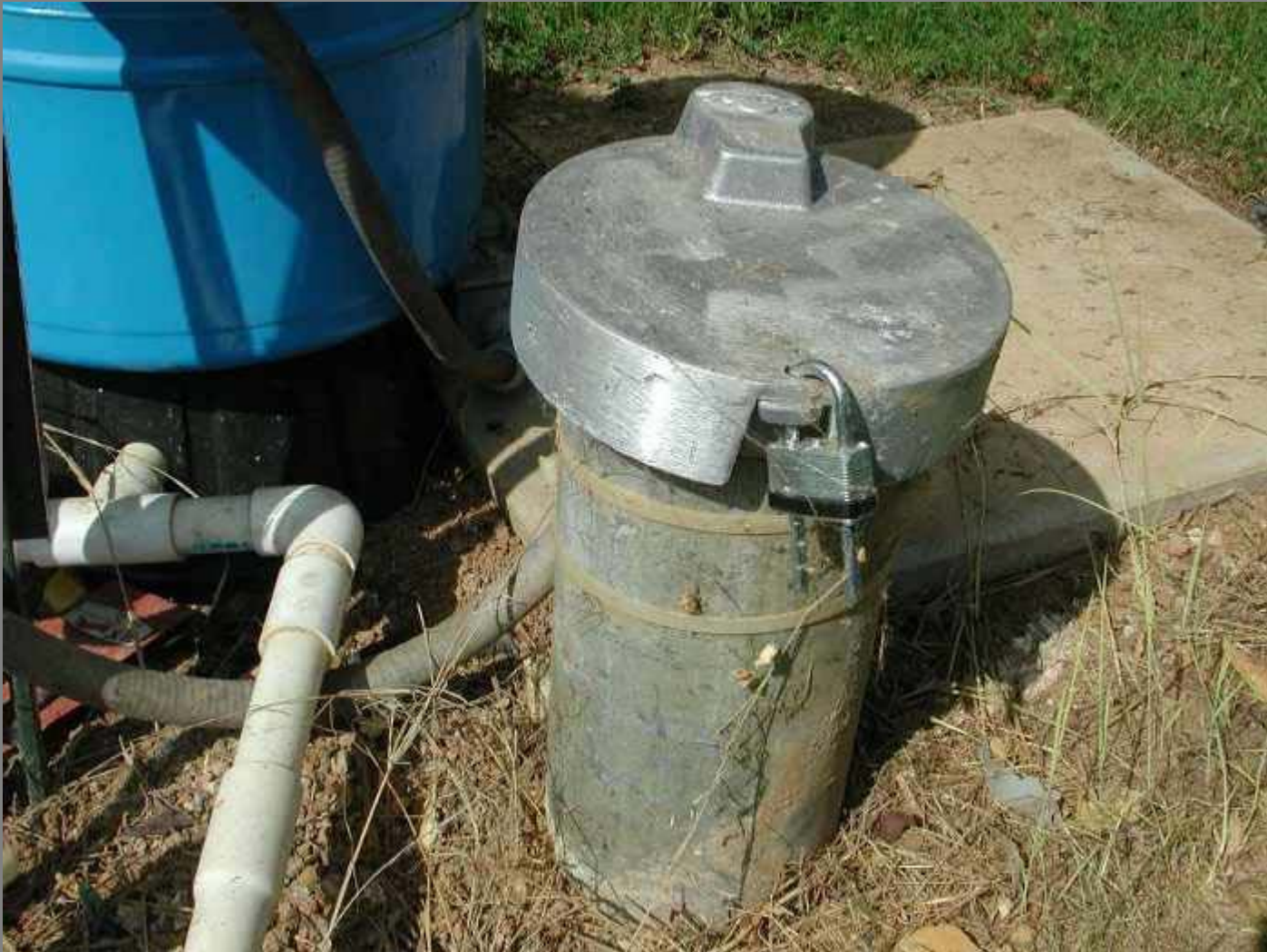
Harry Holt's padlocked contaminated well
